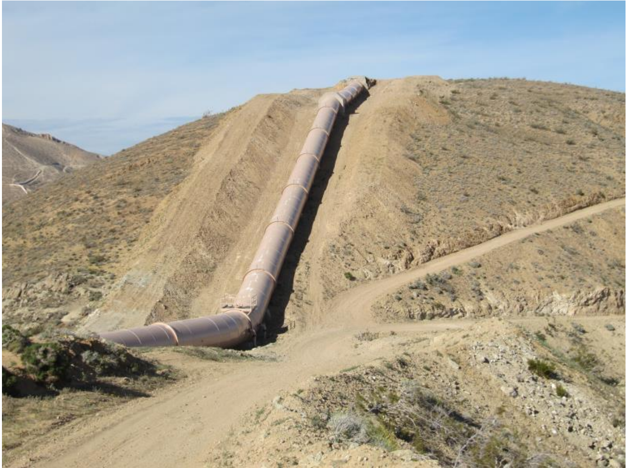
Caption: Los Angeles Aqueduct siphon at Red Rock Canon. From https://venturacountytrails.org/RecentPhotos/2015-03-25RedRockCynSP/IMG_0458_jpg.html accessed Feb. 11, 2024.
